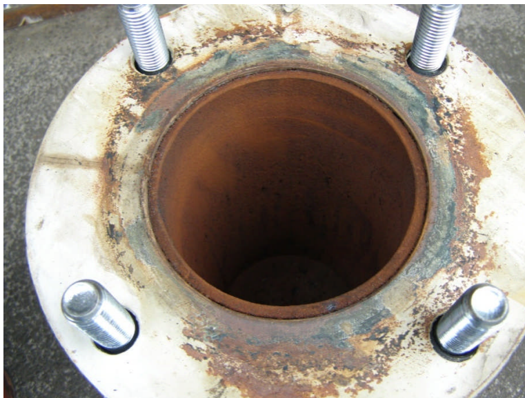
Figure 27 Downdraft Gasification (Food and Paper and Card) Cooler 1 – Rust
